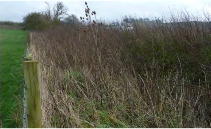
Boundary No.2 (Fence) With Overgrown Ditch on Its Southern Side
